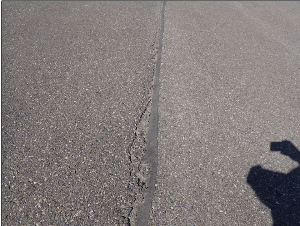
AP-01-01: L&T Cracking
