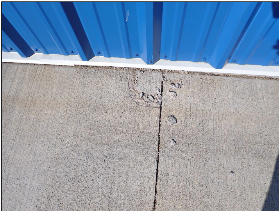
AP-02-02: Corner Spalling
