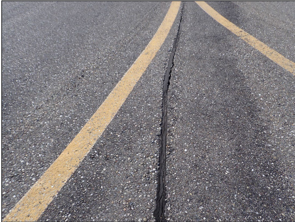
TW-01-05: L&T Cracking
