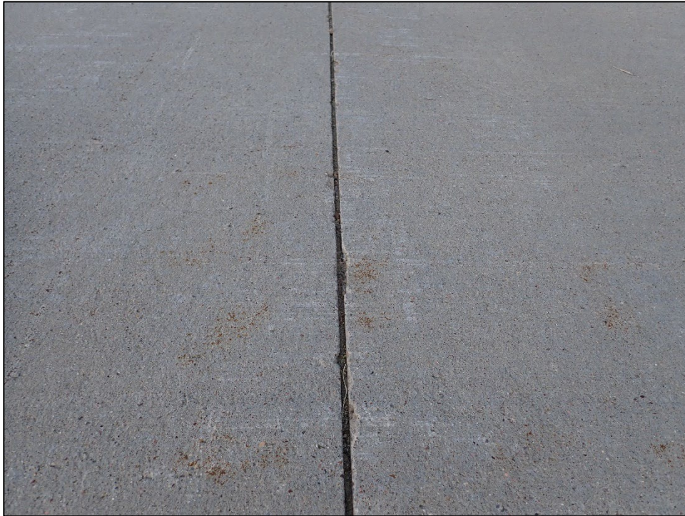
AP-02-03: Joint Seal Damage
