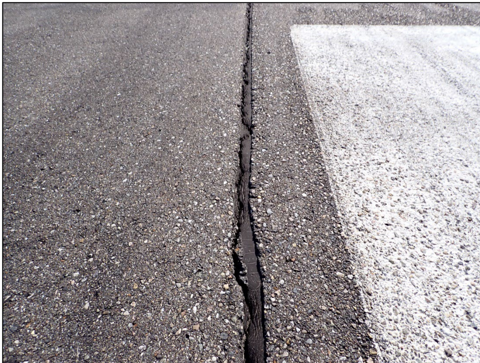
RW13-01-05: L&T Cracking
